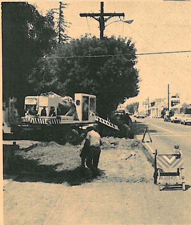
HYNIE WILLIAMS WORKING A DIRT TAMPER ALONG MAINE STREET. THEY ARE REDOING PART OF THE INTERSECTION AND AS USUAL, THEY ARE MAKING A BIG "MESS." (Staff Photo)
